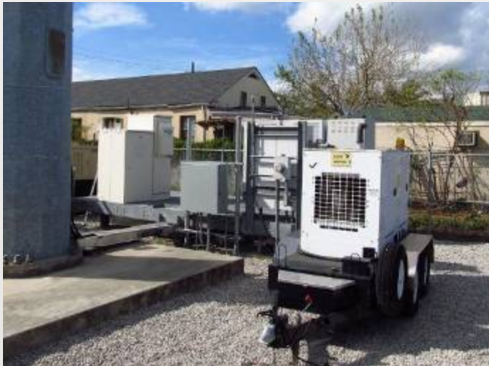
Site with a fuel cell powered by a diesel genset
