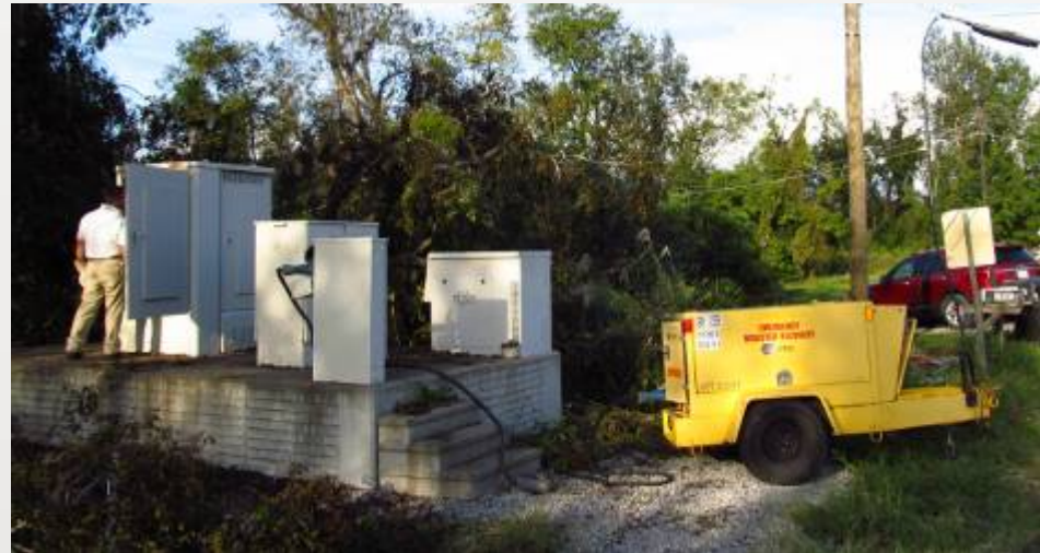
Site with a natural gas generator powered by a diesel genset
