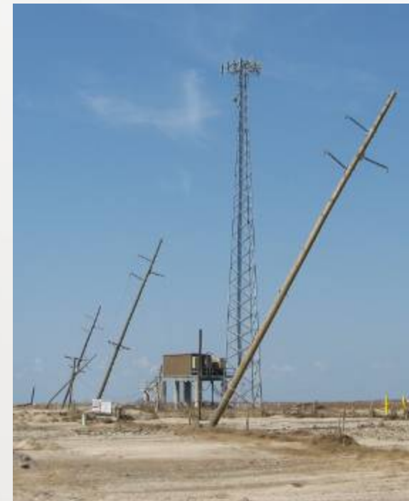
Cell site with a standby diesel genset after Hurricane Ike
