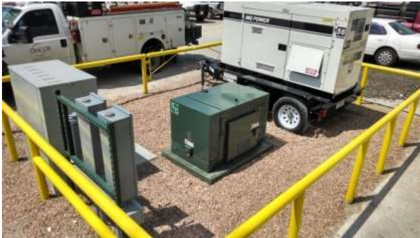
Oncor Initial Installation at Oncor Facility
