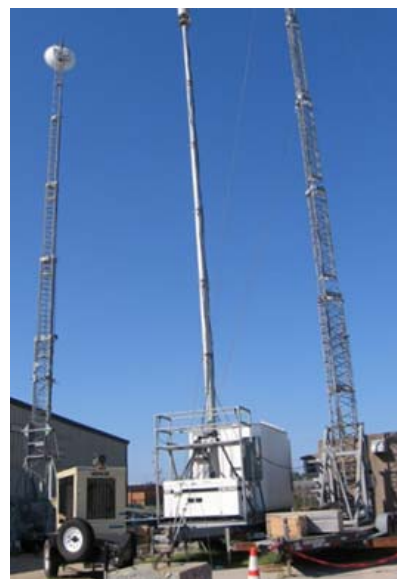
Fig. 13. Sprint-Nextel's COW (middle of the image) and portable transmission site.
