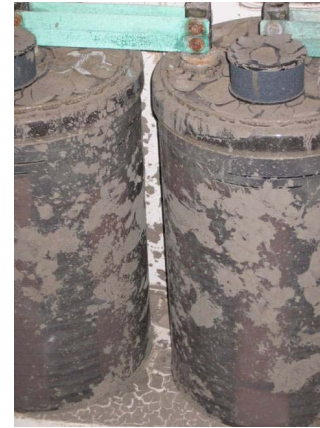
Fig. 2. Batteries damaged due to water immersion.
