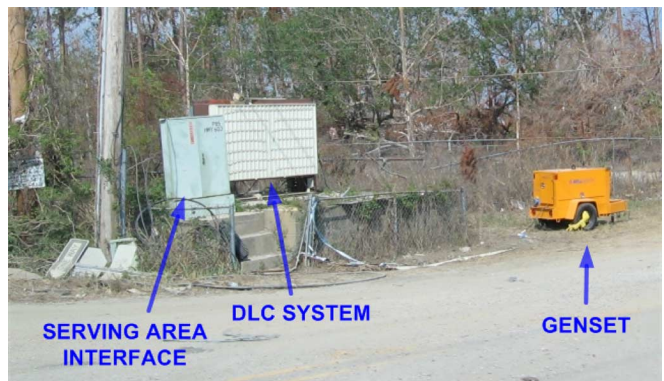
Fig. 9. DLC system providing telephony service to Bay St. Louis CO area subscribers fed with a portable generator deployed after the storm.
