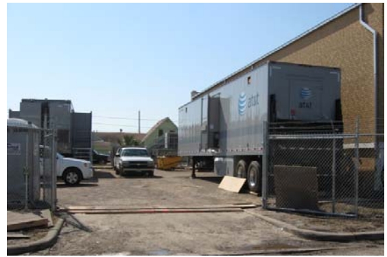
Fig. 13. Switches on wheels behind Sherwood central office.
