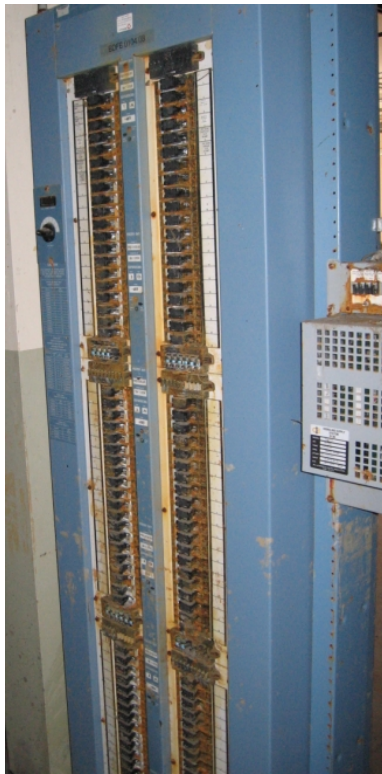
Fig. 4.4. Transmission-system power-distribution frame showing corrosion caused by immersion in sea water
