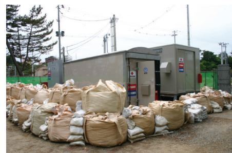
Fig. 23. Shelters with switching equipment used to restore service to Shichigahama CO. Its original building was displaced 500 m by the tsunami.
