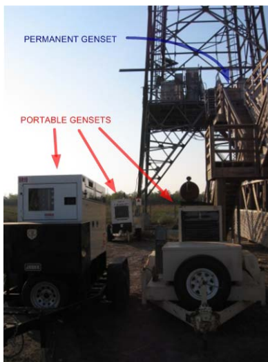
Fig. 15. Cell site in the Irish Bayou, LA with 4 gensets.
