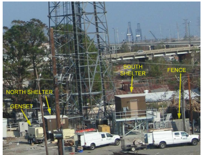
Fig. 14. Cell site in New Orleans with two indoor and two outdoor base stations. The south shelter did not flood.
