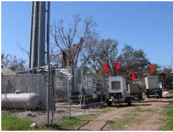
Fig. 14. Cell site in Biloxi, MS where 4 portable gensets, indicated with arrows, were deployed. Another stationary generator not shown in the picture was also installed at the site.
