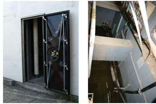
Fig. 14. a) Left: A water tight door in Kamaishi CO. b) Right: Cable entrance facility in Nobiru CO (as seen from the top).
