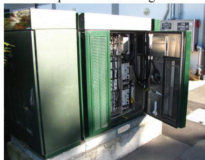
Fig. 10. A minicell base station cabinet showing the door heat exchanger.
