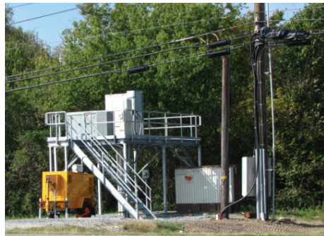
Fig. 5. A new DLC RT with a permanent genset installed on a platform after Hurricane Katrina next to another DLC RT installed on the ground before Hurricane Katrina.
