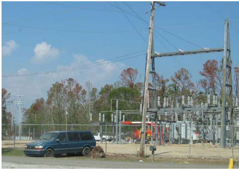
Fig. 8.6. Substation in Waveland, MS
