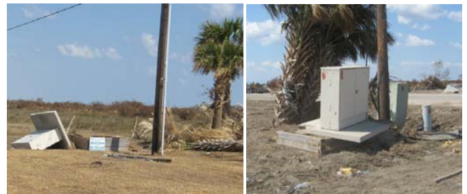
Fig. 15. Two damaged SAIs in the Bolivar Peninsula.
