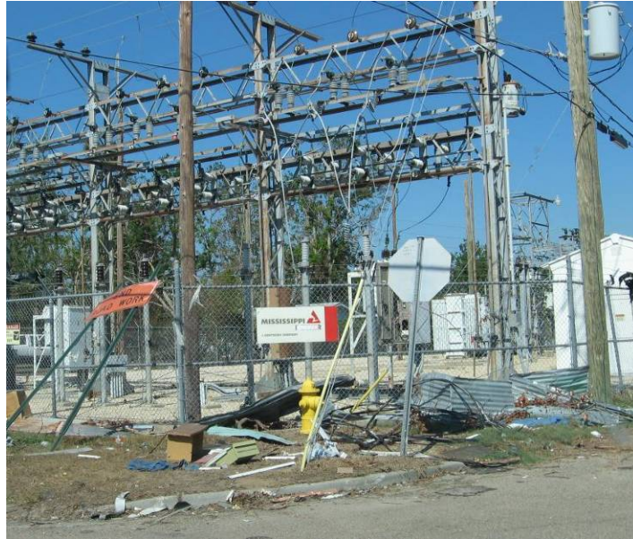
Fig. 8.9. Mississippi Power substation in Biloxi, MS
