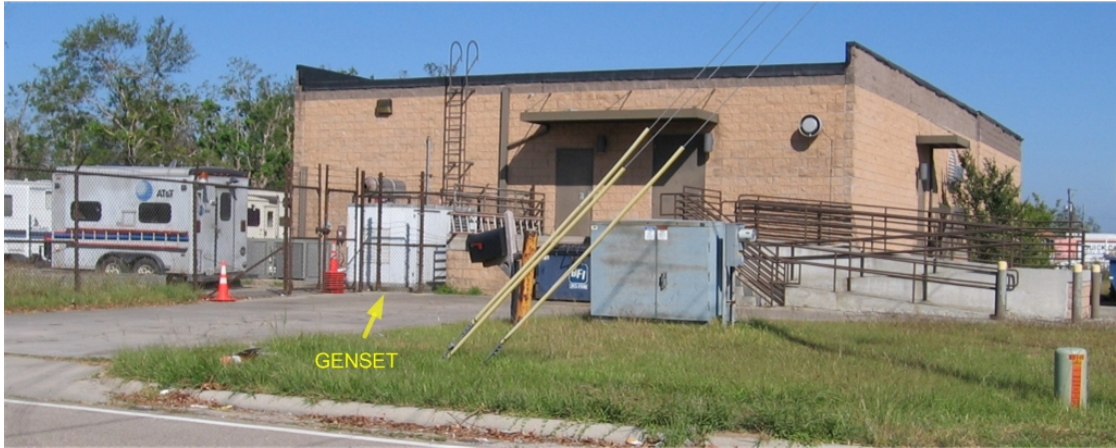
Fig. 5.79. AT&T regeneration site in Gulfport, Mississippi
