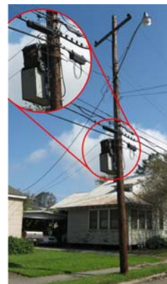
Fig. 8. A portable camping genset on top of a CATV pole-mounted UPS in the town of Plaquemine, Louisiana, after Hurricane Gustav.
