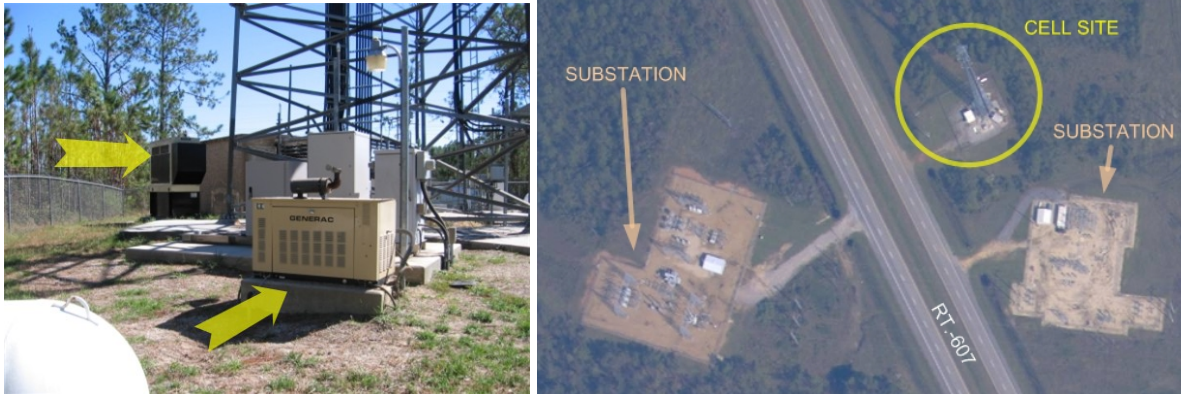
Fig. 6.54. Cell site on Route 607, off I-10 showing two of the three gensets with yellow arrows. Aerial view [6]
