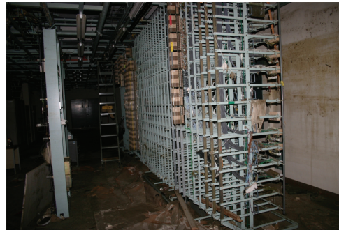
Figure 5. Main distribution frame of a central office that suffered both earthquake shacking and tsunami waves.
