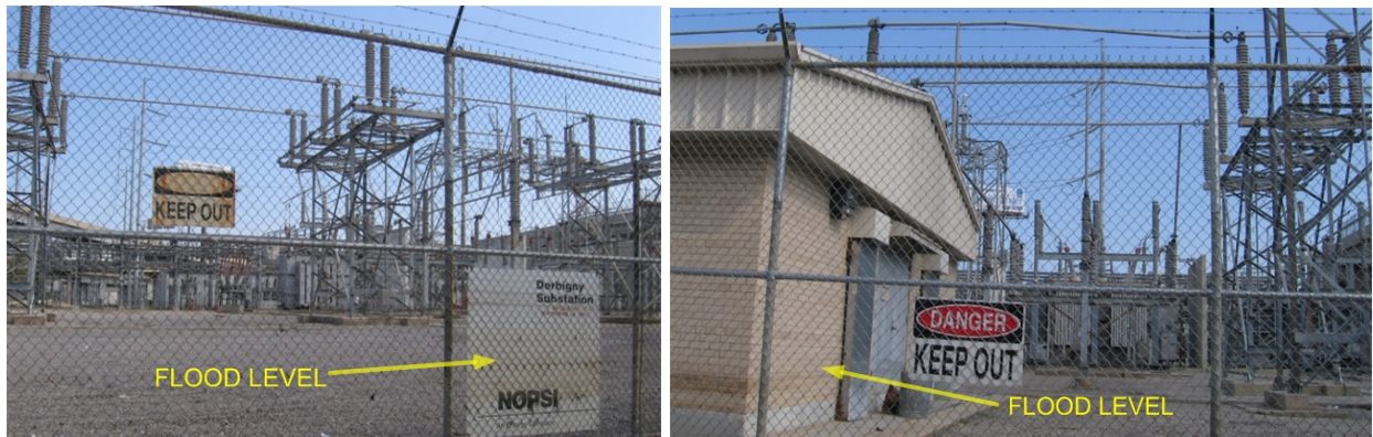
Fig. 8.7. Debirgny Substation near Louisiana Superdome in New Orleans
