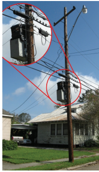
Fig. 9 Genset on top of a pole-mounted CATV UPS after Gustav
