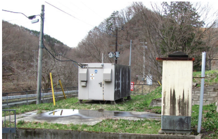
Figure 2. A small remote switch located 20 km east south-east of Morioka.
