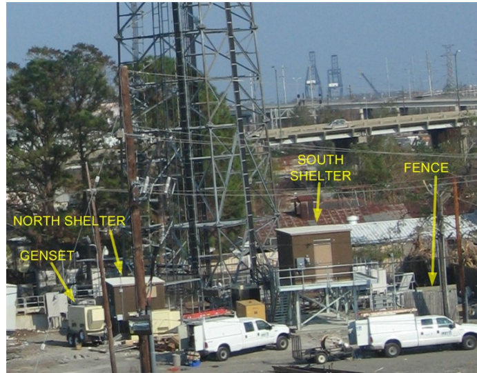
Fig. 6.51. Cell site northeast of downtown New Orleans
