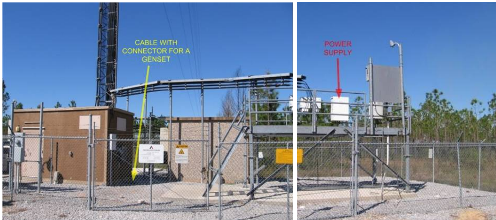
Fig. 6.55. Cell site located at the intersection of Routes 90 and 607
