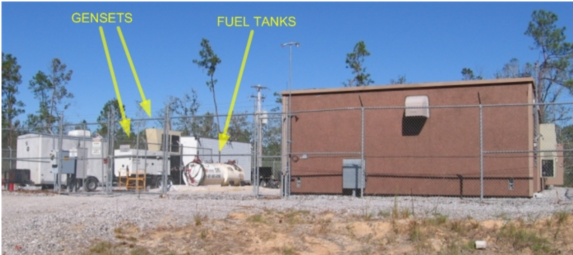
Fig. 5.81. Level3 Communications transmission site south of Pearlington, Mississippi
