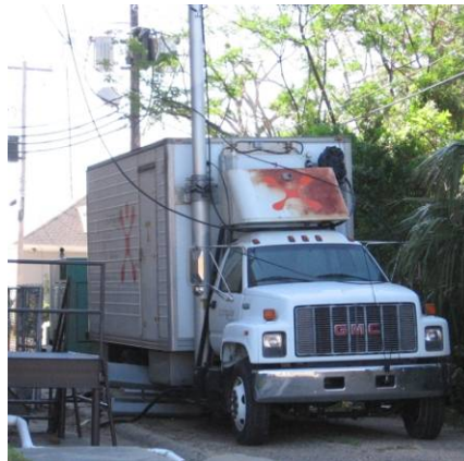
Fig. 6.66. COW behind BellSouth Gulfport CO
