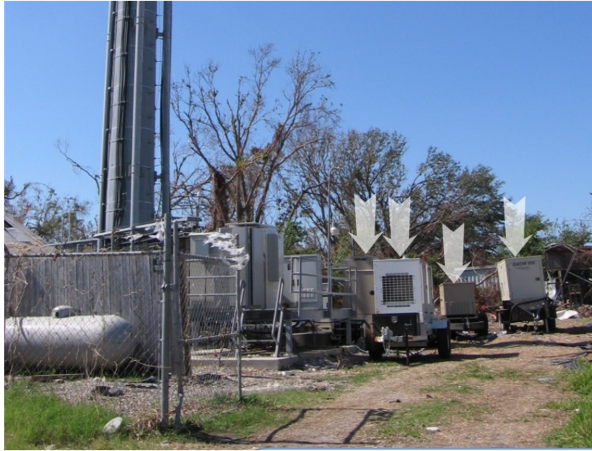
Fig. 6.27. Cell site in Biloxi, MS
