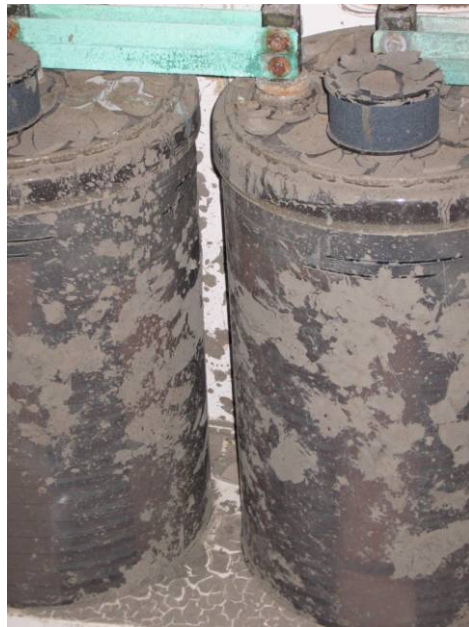
Fig. 4.7. Detail of two battery cells covered in mud. The green-colored interconnection bar is corroded copper.
