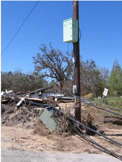
Fig. 17. An undamaged CATV UPS mounted on the pole and a destroyed CATV UPS installed on the ground.
