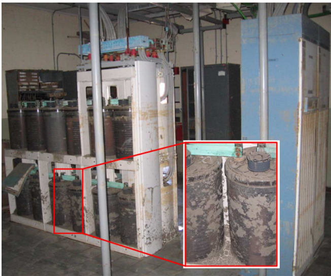
Fig. 2. Interior of a destroyed communications center. The power plant batteries (left and detail) and rectifier cabinets (right) are covered in mud.
