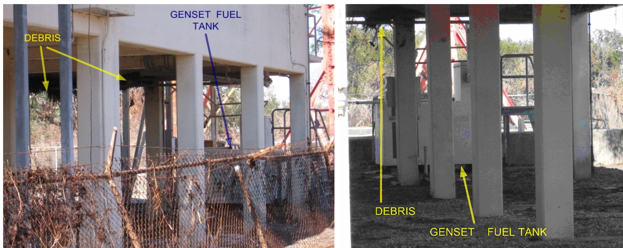
Fig. 5.44. Point A La Hache CO genset fuel tank.
