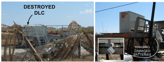
Fig. 1. Destroyed DLC RTs by Hurricane Ike.
