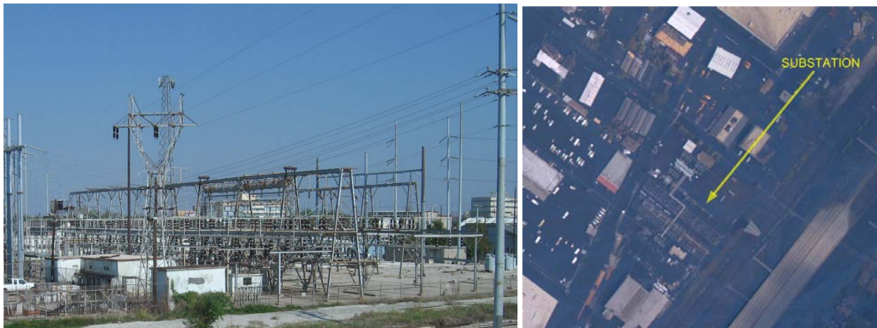
Fig. 8.8. Substation northwest of downtown New Orleans. Aerial view on the right taken on August 31, 2005 [5]
