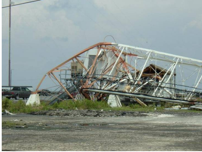
Fig. 6.37. Fallen Tower in Leeville, LA [36]
