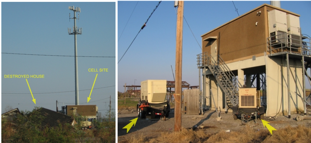
Fig. 6.42. (a) General view of the north cell site in Irish Bayou, (b) Closer view of the same site with two portable generators indicated by yellow arrows
