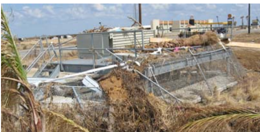
Fig. 2. A DLC toppled and destroyed by Ike's storm surge.
