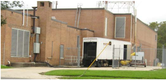
Fig. 9. A large portable generator outside Goodwood central office in Baton Rouge, Louisiana, less than a week after Hurricane Gustav.
