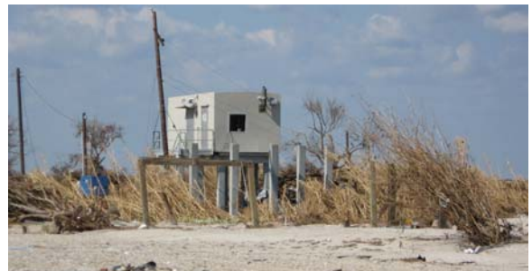
Fig. 5. Cameron Communications site affected by Ike.
