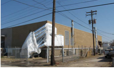
Fig. 12. AT&T's Sherwood CO after Hurricane Ike.
