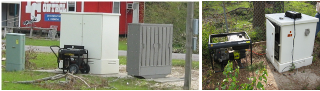
Fig. 6. DLC powered by small gensets. The one on the right failed.
