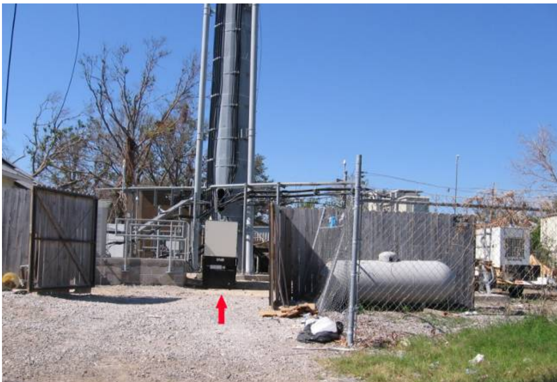
Fig. 6.26. Cell site in Biloxi, MS
