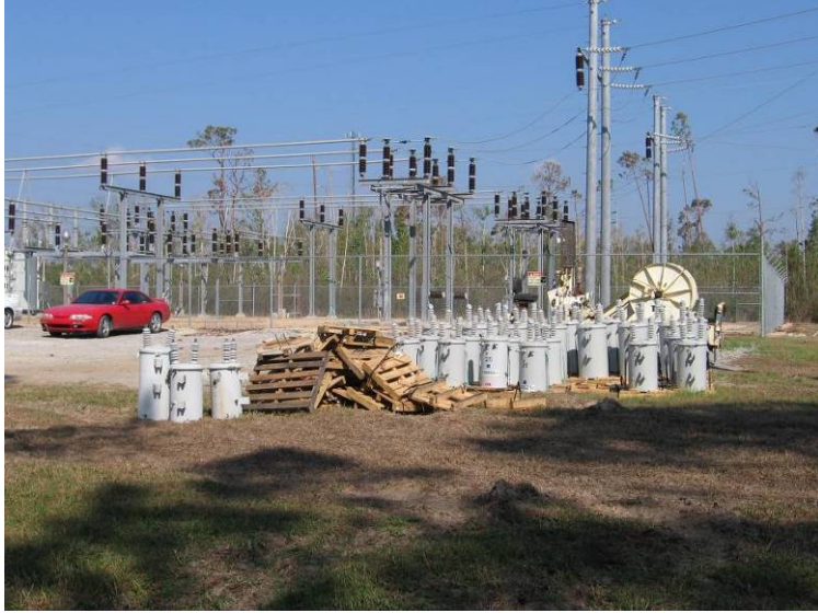
Fig. 8.12. Staged distribution transformers
