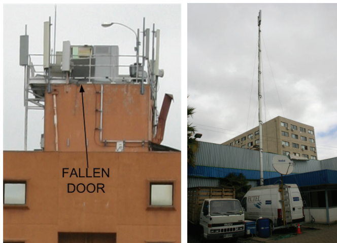
Fig. 9. a) Right: A damaged base station in Curico and b) Left: the COW likely used to restore service in its area. Notice the satellite link in the COW. Stations located on building rooftops needed to be relocated because of the severe damage suffered by the building where they were installed.
