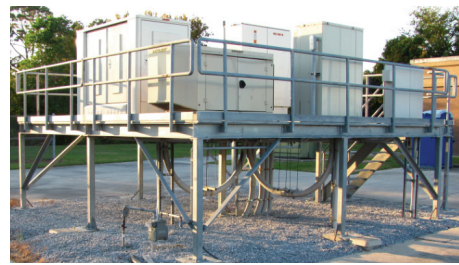
Fig. 4. A DLC RT with a natural gas genset located outside St. Bernard CO destroyed by Hurricane Katrina.
