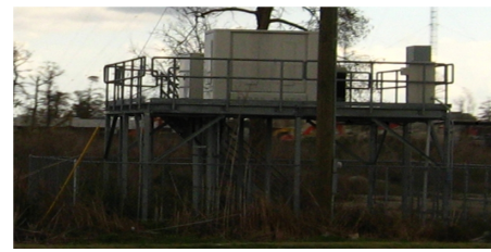
Fig. 2. DLC cabinet on an elevated platform near New Orleans.
