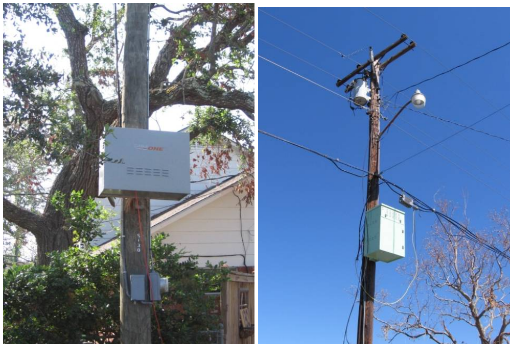
Fig. 7.10. Pole-mounted CATV UPS
