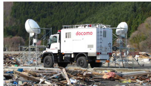
Fig. 21. An Emergency microwave transmission site in Otsuchi.
