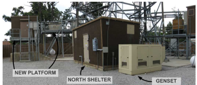
Fig. 15. Photo taken in July 2008 showing a part of the same cell site in Fig. 14 with some improvements but also some equipment around and inside the north shelter below the flood plane.
