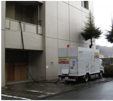
Fig. 11. Miyako CO powered by a mobile generator.
