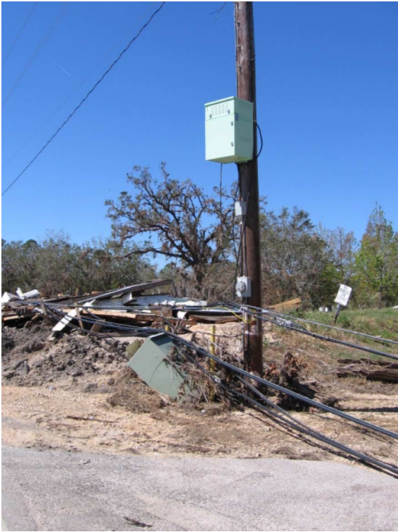
Fig. 11. Undamaged CATV UPS mounted on the pole and a destroyed CATV UPS installed on the ground.
