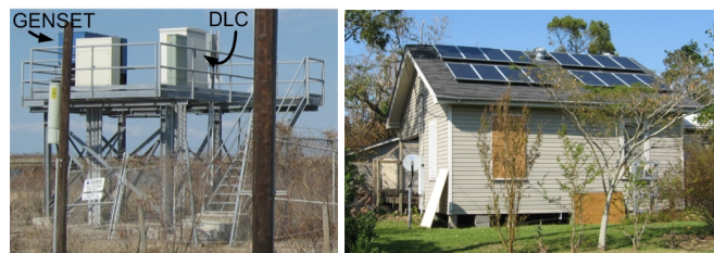
Fig. 10. (a) Left: DLC platform with a permanent diesel genset. (b) Right: House with rooftop-mounted PV modules in Smith Point, TX.
