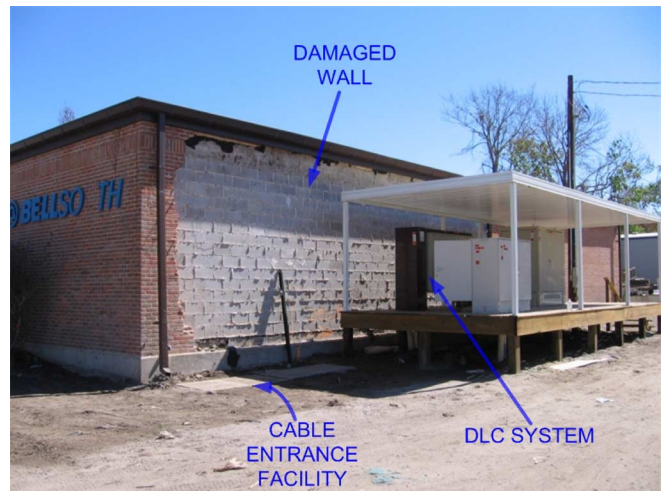
Fig. 8. Pass Christian CO showing the DLC system used to replace the destroyed switch.
