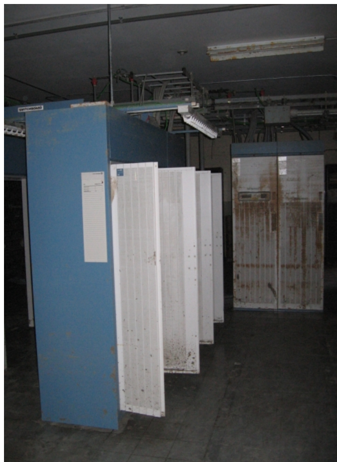
Fig. 4.3. Part of the switch on the left and two rectifier bays on the right
