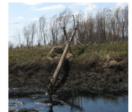
Pole failure mode #1: Extreme wet soil
