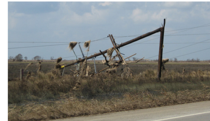
Pole failure mode #1: Broken pole due to high winds
