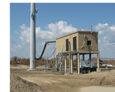
Camping genset on pole (inadequate)
