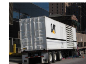
Power outages: Gensets
