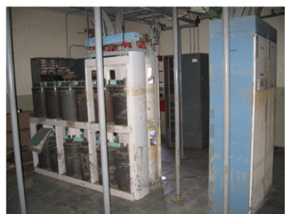
Destroyed communications center
