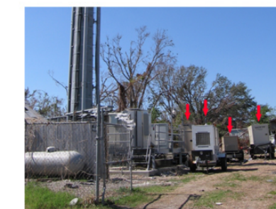
Multiple gensets at each cell-site
