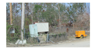
Digital loop carrier with genset
