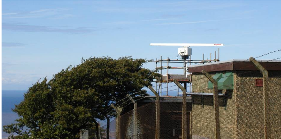
Fig 24 : BHP Billiton radar at Gwaenysgor
